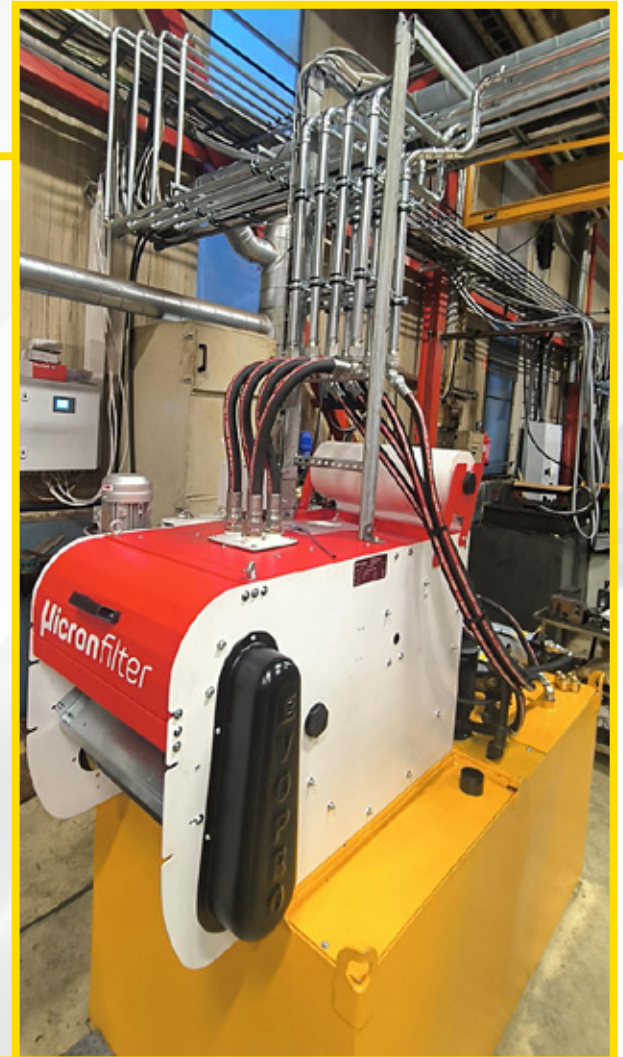
On the right: Evotech Pro 500 supplied by Tekupit to Urjala Works. Tekupit also provided the system's transfer pumps and the control box that manages the operation of the entire system.
