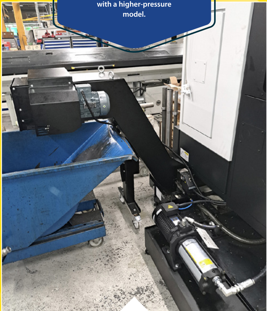
19.5 bar upgrade set, installed
